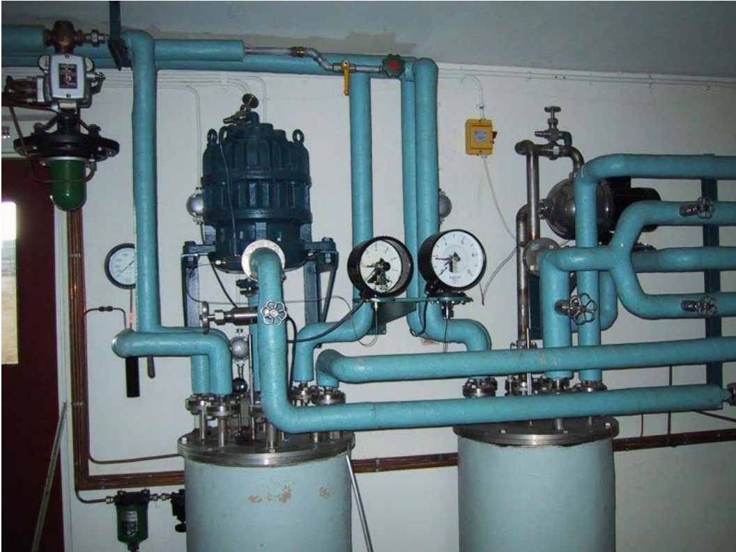
Figure 9 Heat exchangers and cooling pumps. The system to the left belongs to the core cooling circuit, the one to the right to the recombiner cooling circuits.
