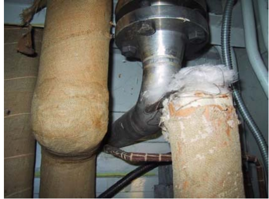
Figure 11 Flange at the bottom of the recombiner
