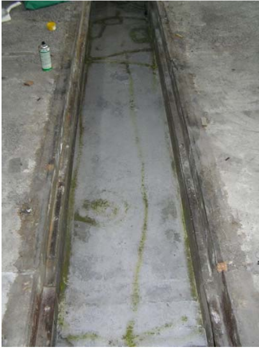
Figure 60 Contaminated parts in the southern channel marked by yellow spray paint
