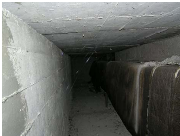
Figure 67 A view into the northern channel with an air heating channel to the right
