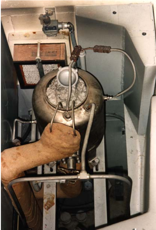
Figure 10 The recombiner seen from above
