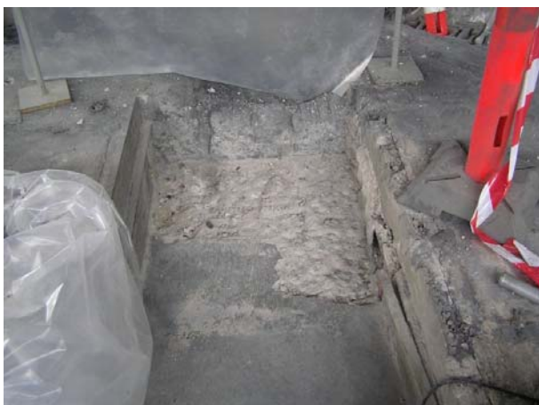
Figure 58 Extent of contamination in the northern channel
