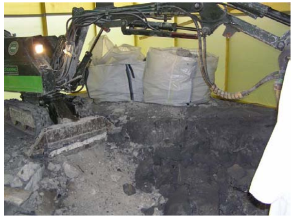
Figure 45 The demolition robot in action. Two big bags with excavated material in the background
