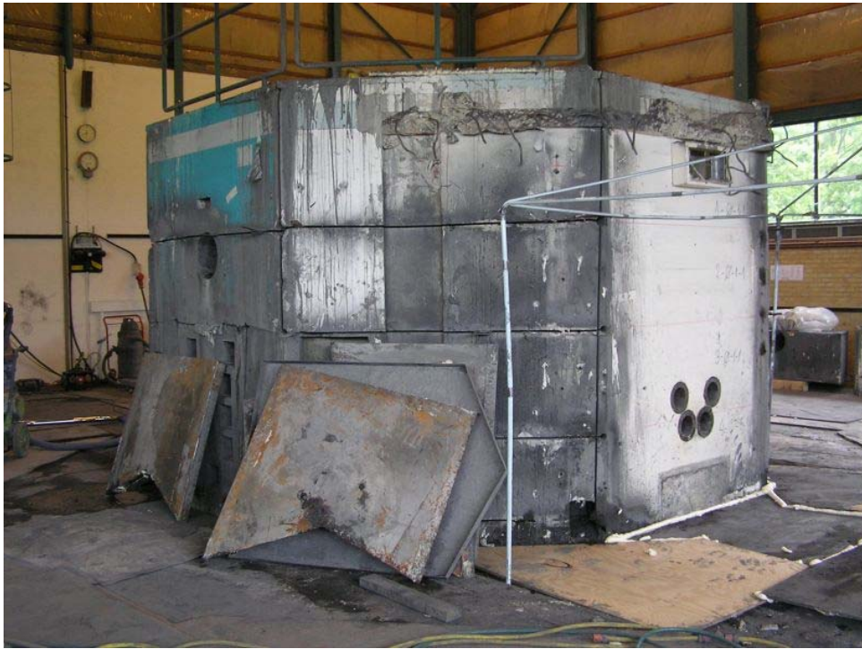
Figure 37 Vertical and horizontal cuts in the reactor block. In the foreground trays used for collecting cutting water.
