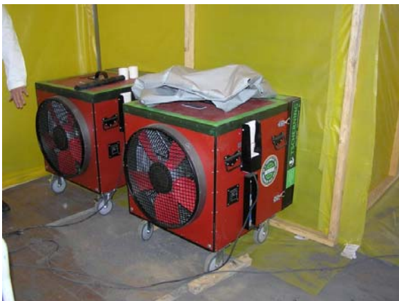
Figure 42 Ventilators with HEPA filters
