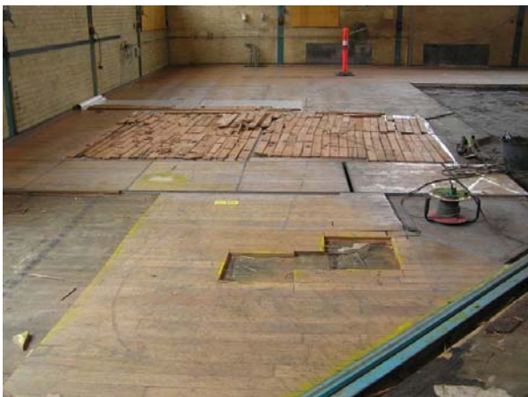
Figure 46 Contaminated parts have been cut out from the wooden floor. In the background a section of floor boards have been taken up.
