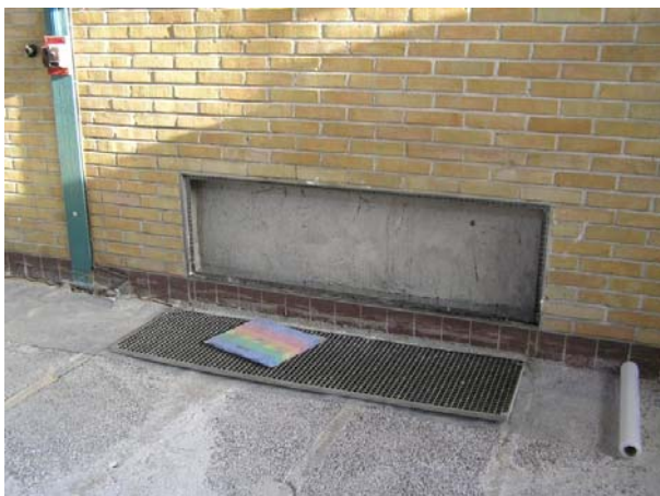
Figure 66 One of the three outlets for the air heating system
